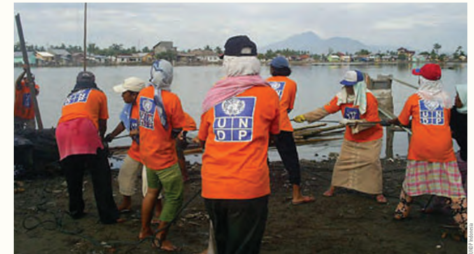
Workers, in Aceh, Indonesia, remove debris after the 2004 Tsunami as part of a UNDP emergency infrastructure rehabilitation project.
