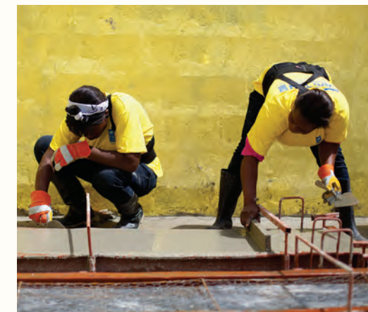
Female construction workers, employed through a UNDP programme repair a house in Haiti.
