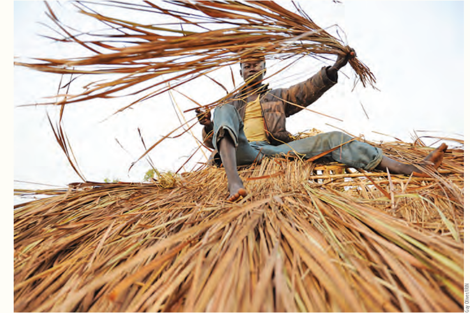
A displaced person from Ngubu camp, the Democratic Republic of the Congo, builds a permanent structure.
